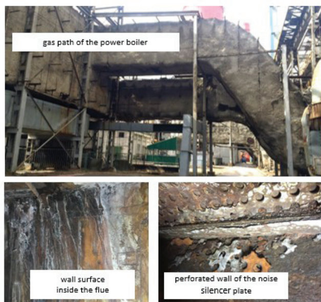
Fig. 1: Corrosion of the metal of the gas path of the boiler under the influence of condensate from flue gases
