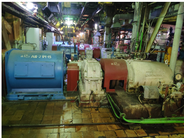
Fig. 5: Photo of high pressure ammonia pump «URACA» in the shop 4 of «KuibyshevAzot» public joint stock company.
